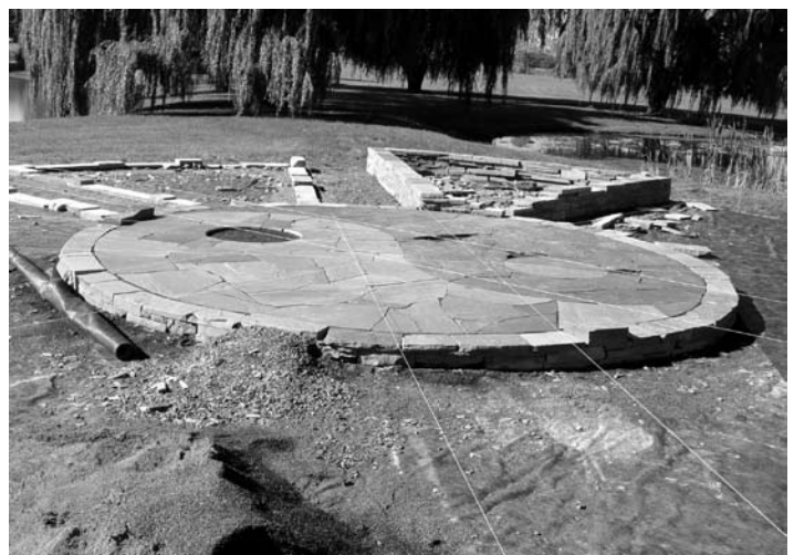
Construction of NYCC's herb garden has begun and is expected to take six to eight weeks to complete. Jerry Fox and Larry McCoach of Against the Wind Stonework in Willet, N.Y. (near Cortland), are building the beds and patio.
